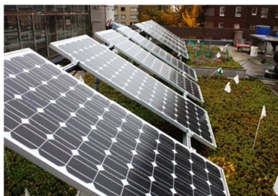
Figure 1. PSU Photovoltaic Test Facility
